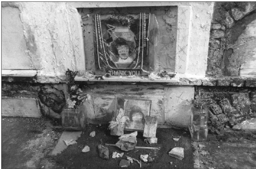
Gravesite of Amanda Carroll, February 23, 1990. X marks are faintly visible on the wall above the vault.
